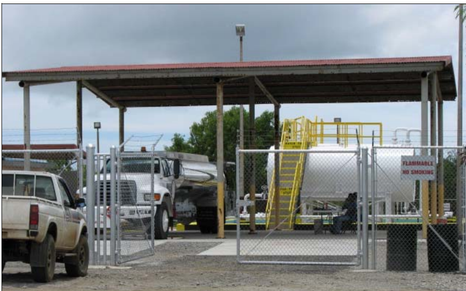
Yap International Airport jet fuel supply facilities repaired and ready to service
